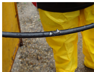
Copper cable damage
