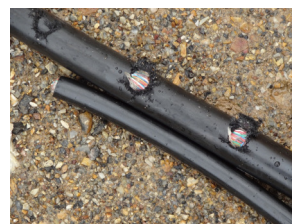
Copper cable damage
