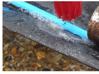
Optical Fibre damage
