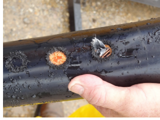
Power Cable Damage
